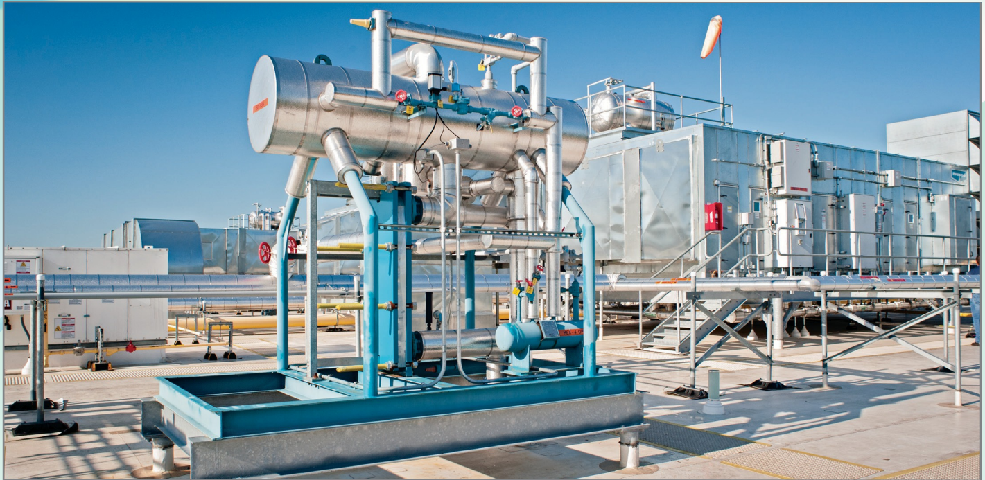
RVS MPC Chiller Package
